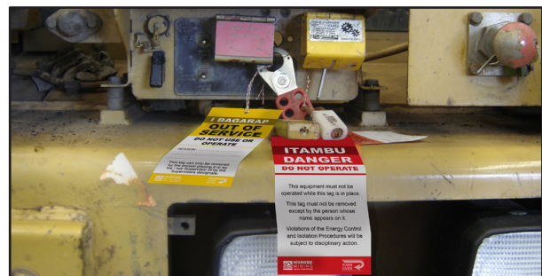
Out of Service Tag and Danger Tag
