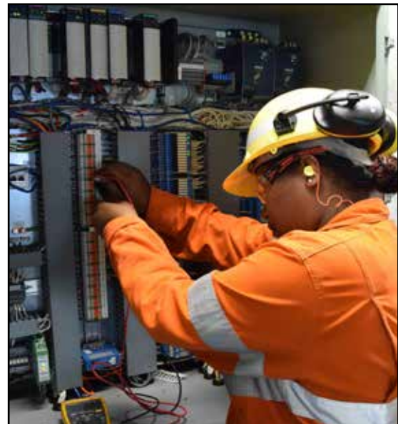
Treat all wires as live unless tested otherwise
